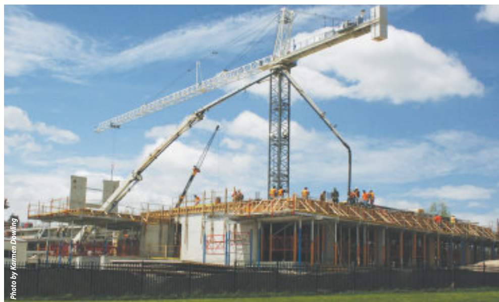
Photo by Karmen Dowling Construction is well underway for the new Ivey building on Western Road. The $100-million project is expected to be complete by March 2011.
